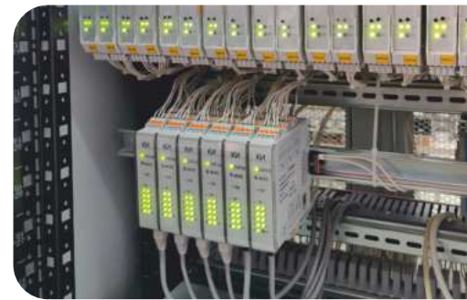
ESSO-ILS tower equipment
