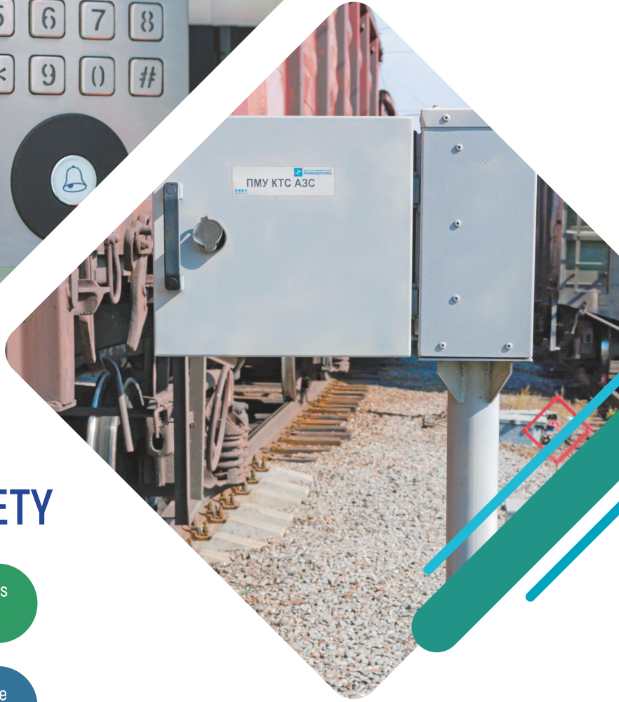
Local control panel
