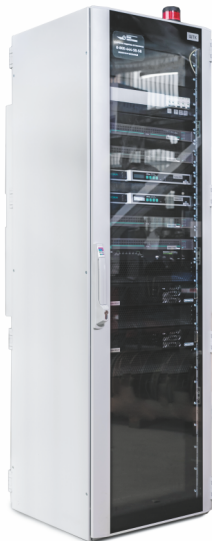
ShTK Telecommunication Cabinet
