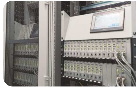
ESSO-M-2 tower equipment
