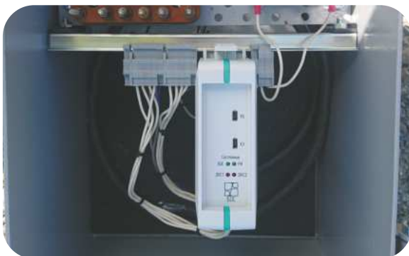
BOS Signal Processing Unit
