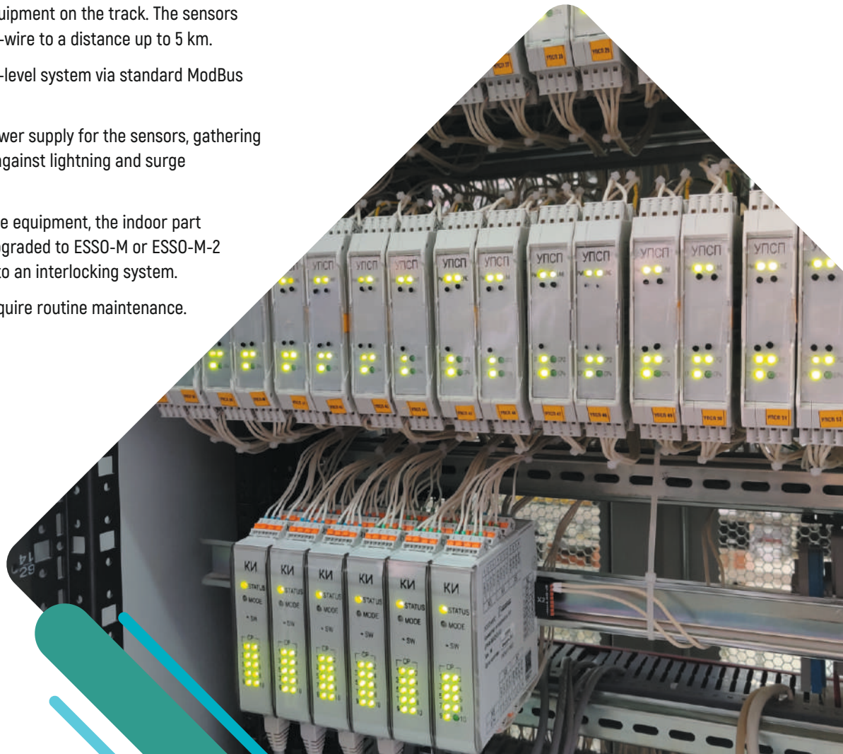
ESSO-ILS Indoor equipment
