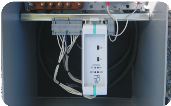
BOS Signal Processing Unit
