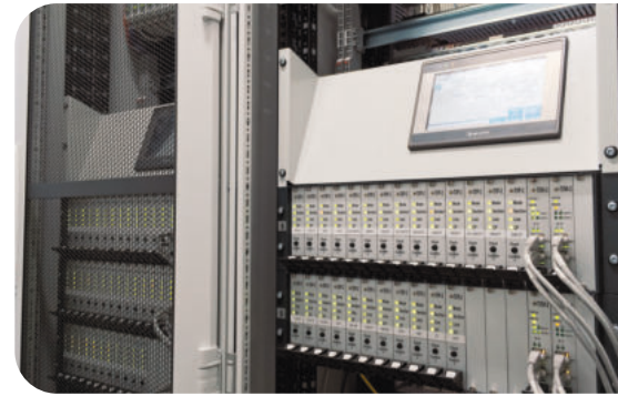
ESSO-M-2 tower equipment
