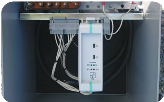
BOS Signal Processing Unit
