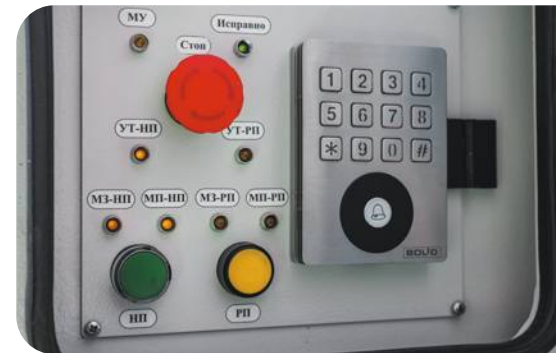
Local Control Panel
