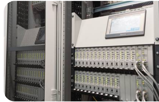
ESSO-M-2 tower equipment
